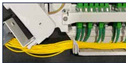
Patchcords guided to the side, protected by front door with label for port identification
